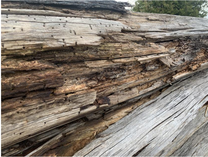
Photo 1: Termite and rot damage on logs
