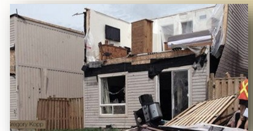
Damage from the Angus Ontario Tornado 2014
