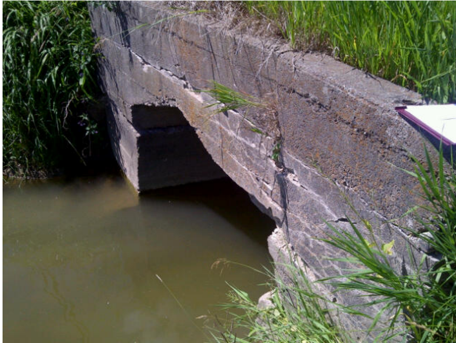
Figure 3 - Structure #2 (CR#25)-External concrete deterioration
