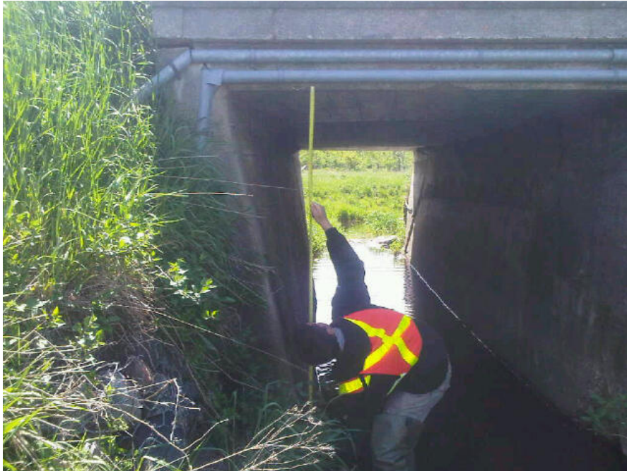
Figure 1 – Structure #1 (CR#9)-Legs sheared from footing and shifting inward (approx.. 600 mm)
