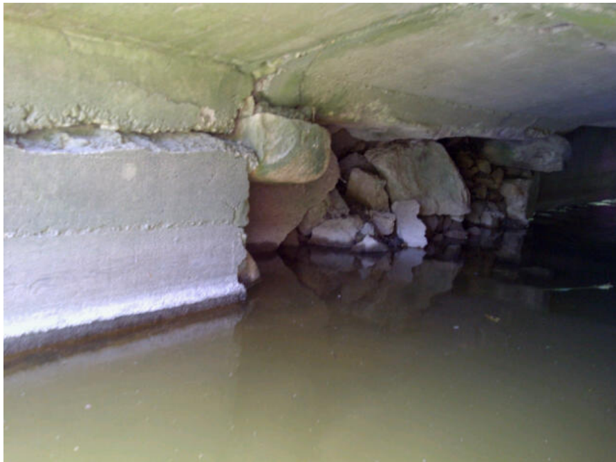
Figure 4 - Structure #2 (CR#25)-Legs shearing from platform and Internal concrete failure
