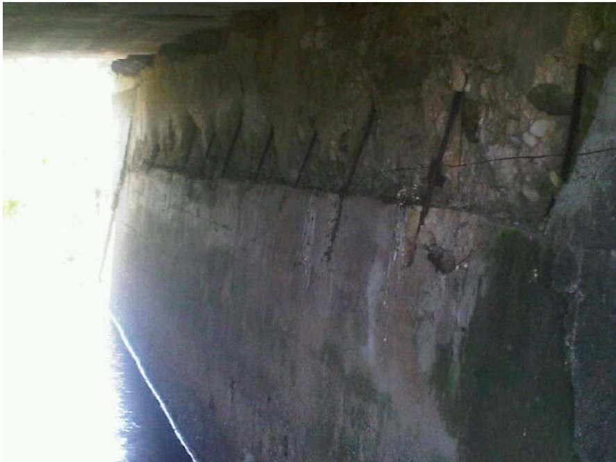
Figure 2 – Structure #2 (CR#9)-Internal concrete failure and exposed steel reinforcing bars
