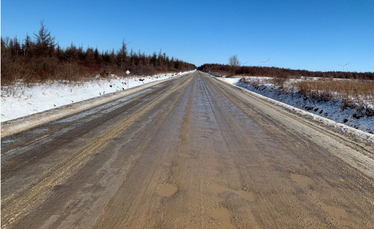
(R3) Dufferin County Road 21 – Reconstruction Project to be Paved with Hot Mix Asphalt
