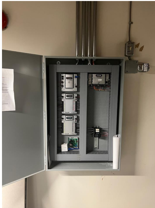
Building Automation System Upgrades
